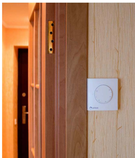
Termostat Electromecanic SEITRON TM 001M in the interior
